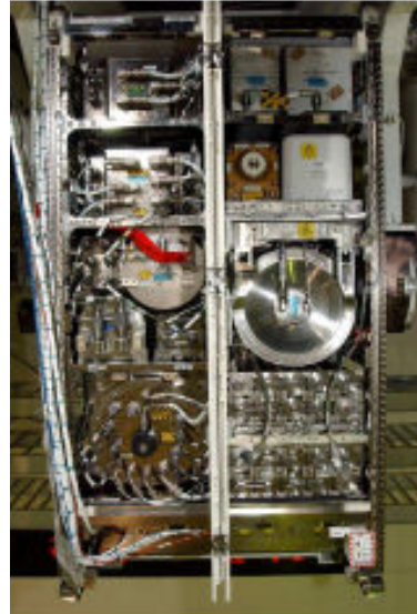
Water Recovery System (WRS) Rack #2
