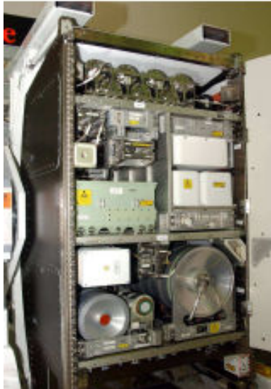
Water Recovery System (WRS) Rack #1
